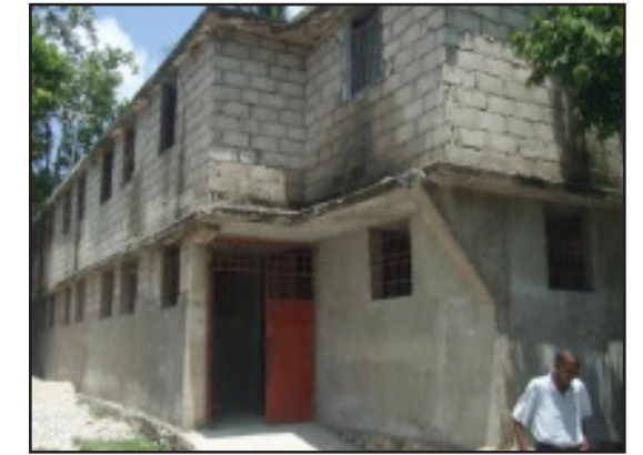
Work done to the EE Training Center in Les Cayes, run by Pastor Banes, EE Haiti Director, stabilized it in preparation for any future earthquakes. This building houses a Vocational Technical Training School and Print Shop.
