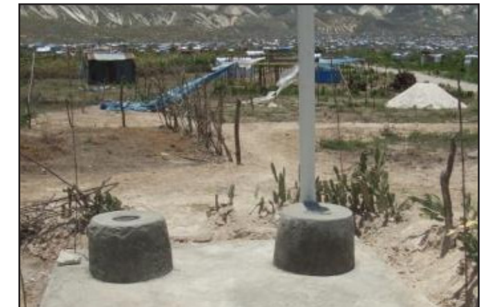
The GSCC team digs down 15 feet and pours the concrete before they leave.
